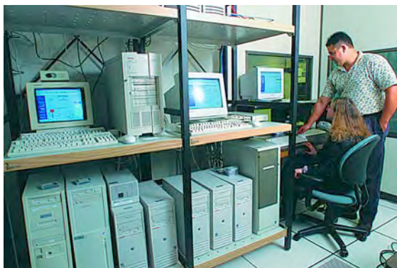
SMART chemWORKS server
