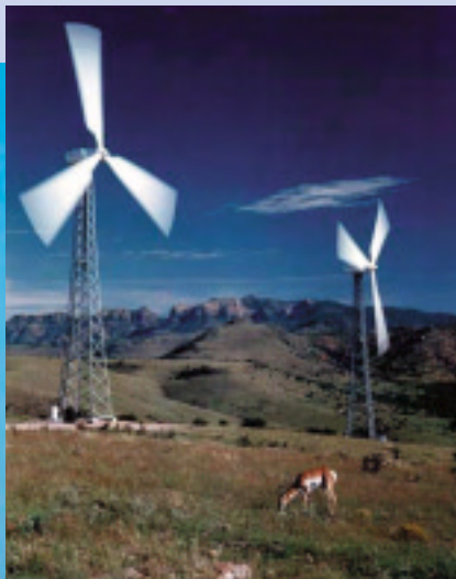
Central and South West: Fort Davis, Texas; twelve 500-kW Zond Z-40A turbines
