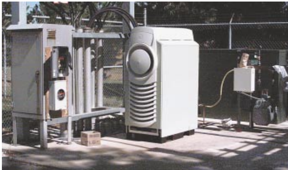
COURTESY, AMERICAN ELECTRIC POWER CO.
