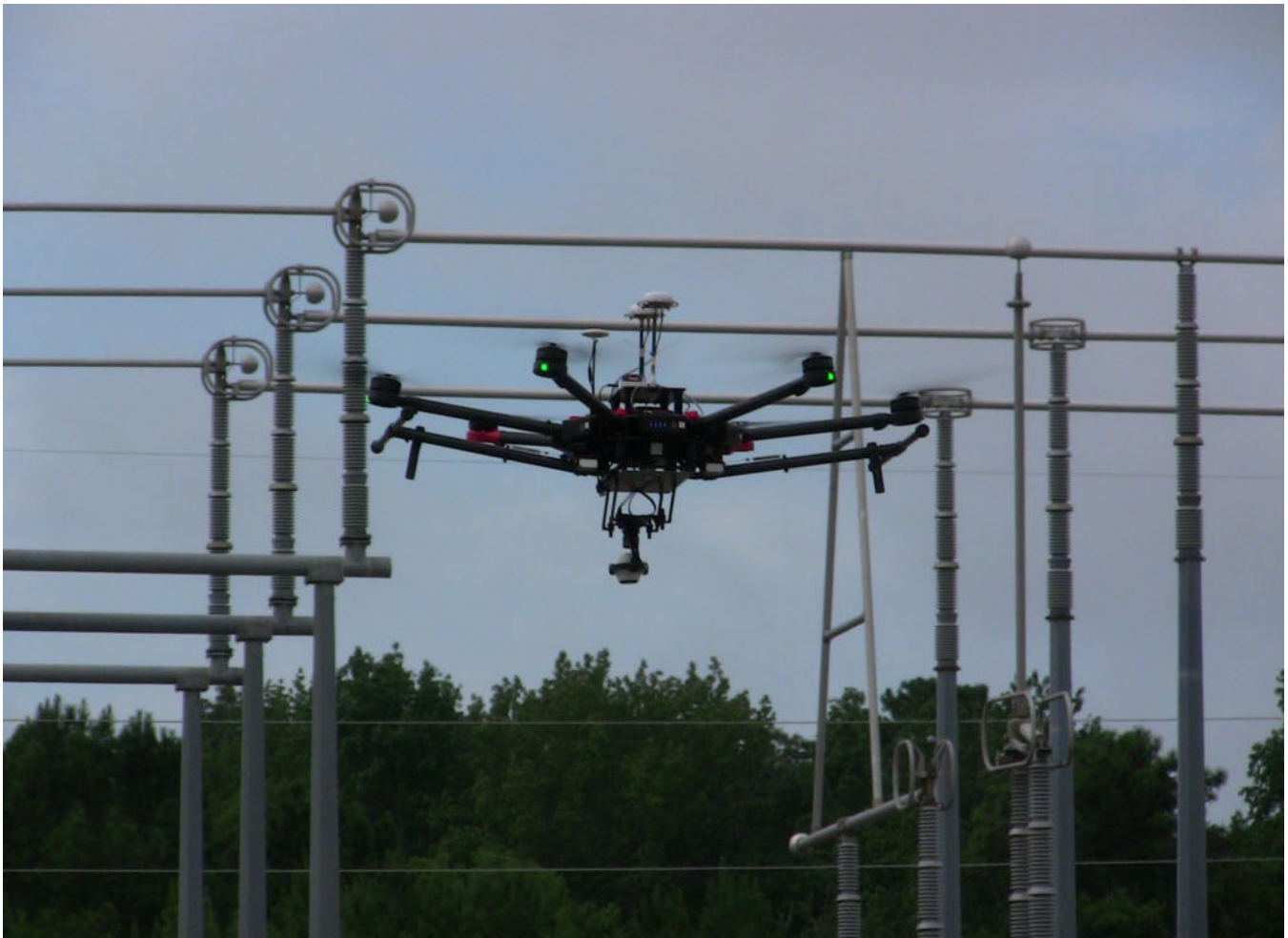
A drone collecting images of substation equipment during an EPRI field test.
