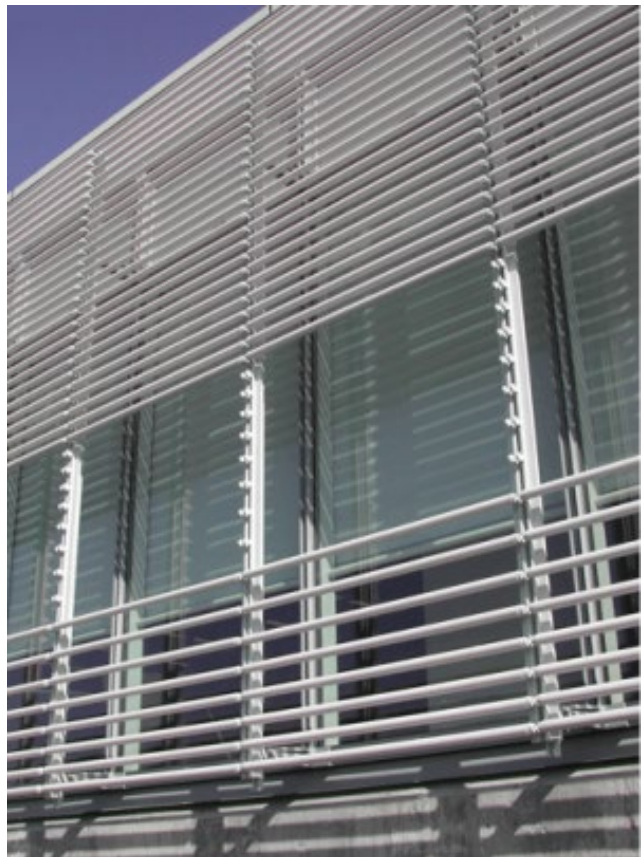
This photo shows part of a full-scale, 5,000-square-foot mockup of the corner of one floor of the New York Times Headquarters Building. Before purchasing the building, the New York Times Company invested in this mockup to test and optimize various window, façade, and lighting technologies—with technical support from Lawrence Berkeley National Laboratory. These include low-emissivity window glazing to reduce winter heat loss and summer solar heat gain, exterior ceramic rods to diffuse daylight, and interior automated roller shades to control glare, daylight, and solar energy. Photo courtesy of Lawrence Berkeley National Laboratory.
