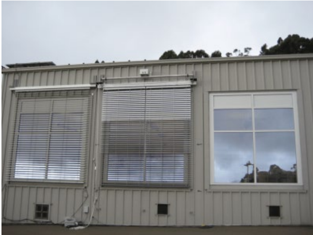
This photo shows testing of shading systems at Berkeley Lab's Advanced Facade Testbed. The room on the left is equipped with an automated external blind system that manages solar heat gain and glare. The center room uses an automated external dual blind system, with a lower portion that controls solar load and glare and an upper portion that redirects daylight inside. The room on the right uses conventional interior manual blinds. The study found that the external systems can reduce cooling loads by 50–85% relative to the conventional blinds. Photo courtesy of Lawrence Berkeley National Laboratory.
