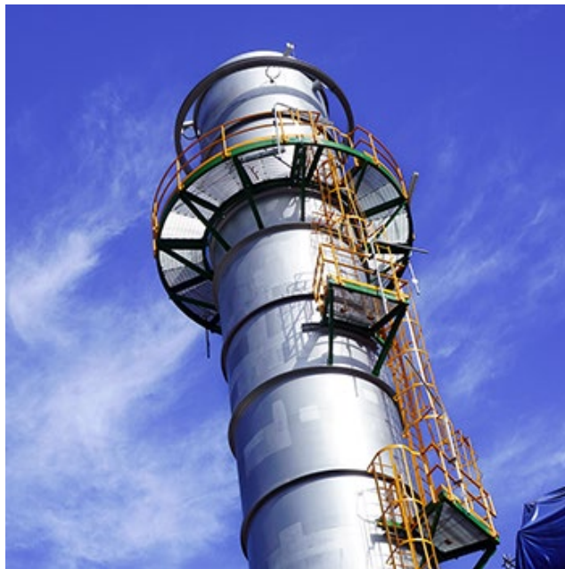
© Adobe/Gas turbine power plant stack
