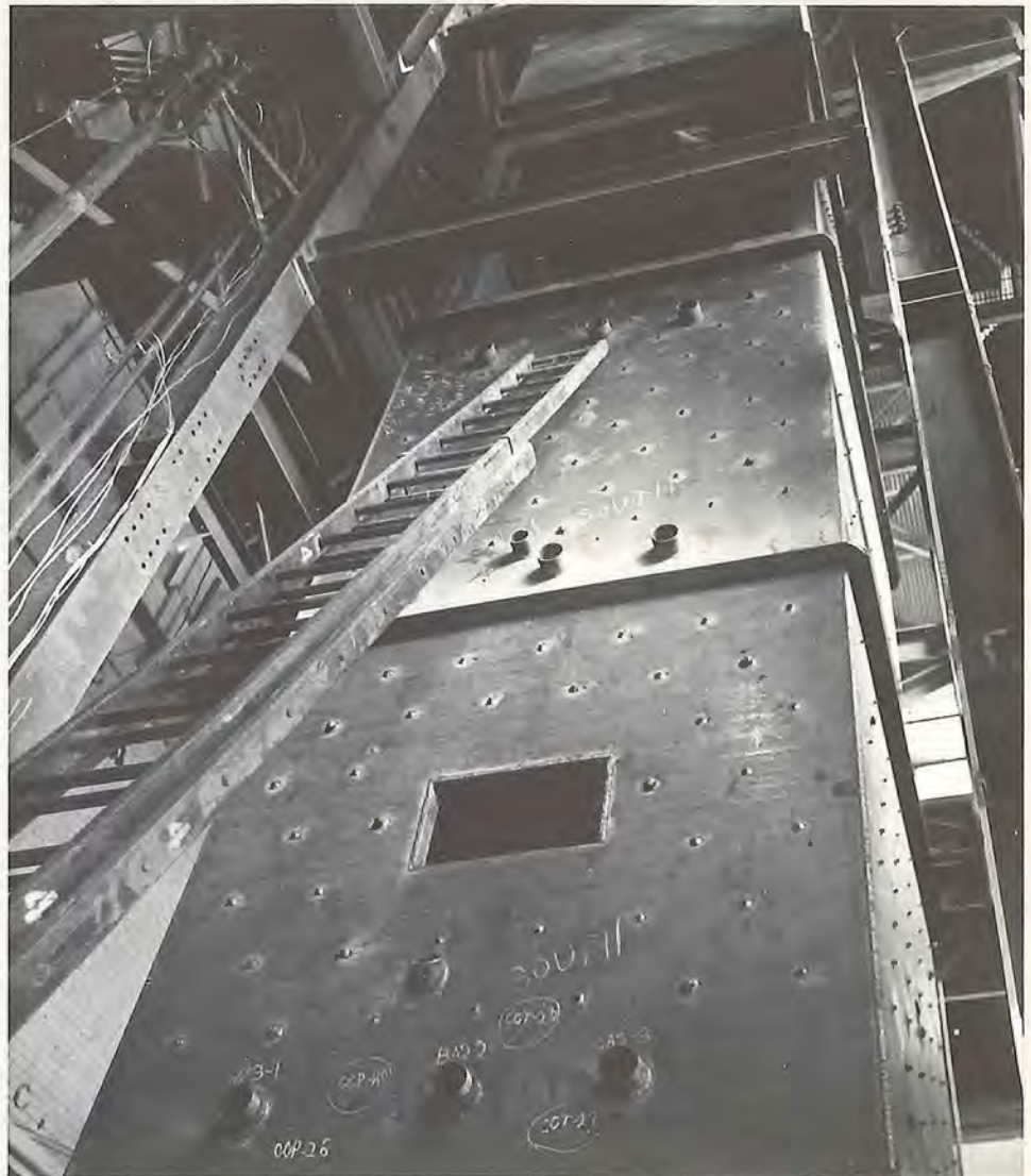
Figure 4 Construction of a 36-ft 2 fluidized-bed development facility will be completed in September.
