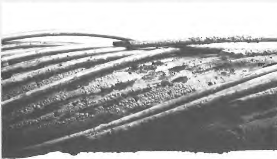
Figure 2 Typical corrosion of concentric neutrals surrounding buried cables.
