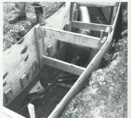
Figure 5 Obstructions, such as might be encountered in urban trenches, are represented in this test of the trench shoring in which the horizontal members (located 0.45 m [18 in] from the bottom of the trench) can be bypassed without difficulty.
