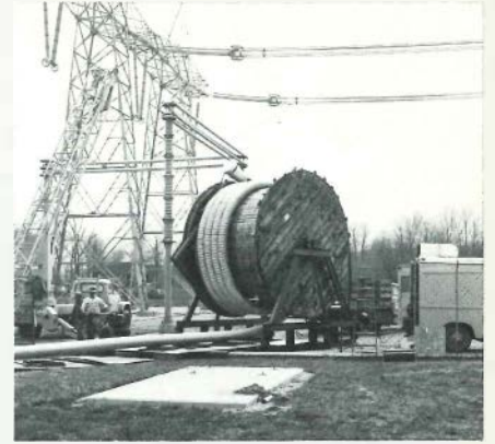
Figure 3 Flexible, gas-insulated cable on reel, shown at the start of the pulling operation at the Waltz Mill facility.
