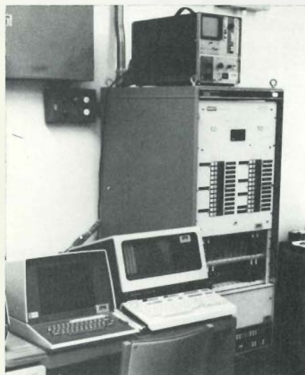
Figure 4 The on-line vibration-monitoring system installed in Northeast Utilities' Millstone-2 nuclear power plant consists of vibration instruments (center right), a digital computer (lower right), an FFT analyzer (upper right), and terminals for operator interface (left).
