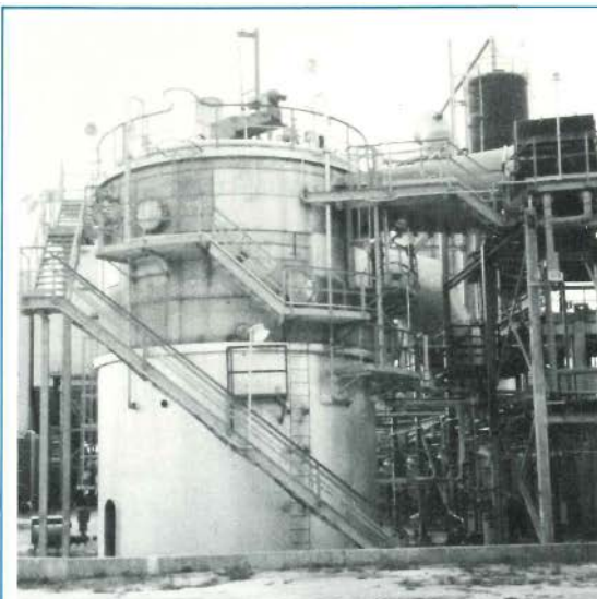
Chiyoda Thoroughbred-121 jet bubbler reactor, part of 20-MW prototype scrubber system at Scholz plant.
