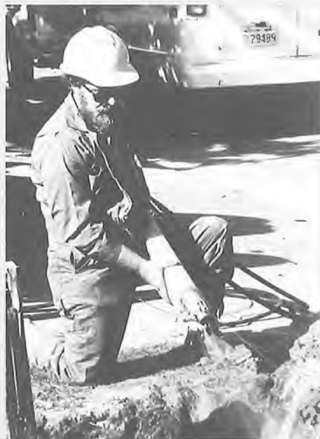
Figure 3 Cable follower with activated jets, ready to be loaded onto a cable. The water jets can be reconfigured to the best advantage for the type of soil being penetrated.
