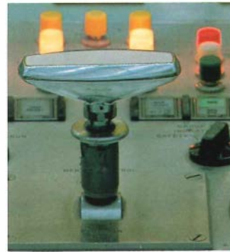
Research on human factors, such as control room design, helps ensure the safe operation of nuclear plants.
