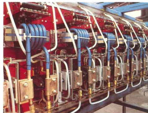
HVDC transmission could soon be an important means of bringing bulk power to congested cities. This compact HVDC converter station prototype is in Queens, New York.
