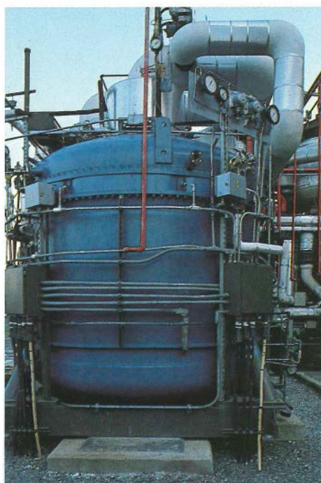
A catalytic steam reformer converts fuel and steam to hydrogen for powering the 4.8-MW fuel cell demonstration in Manhattan.
