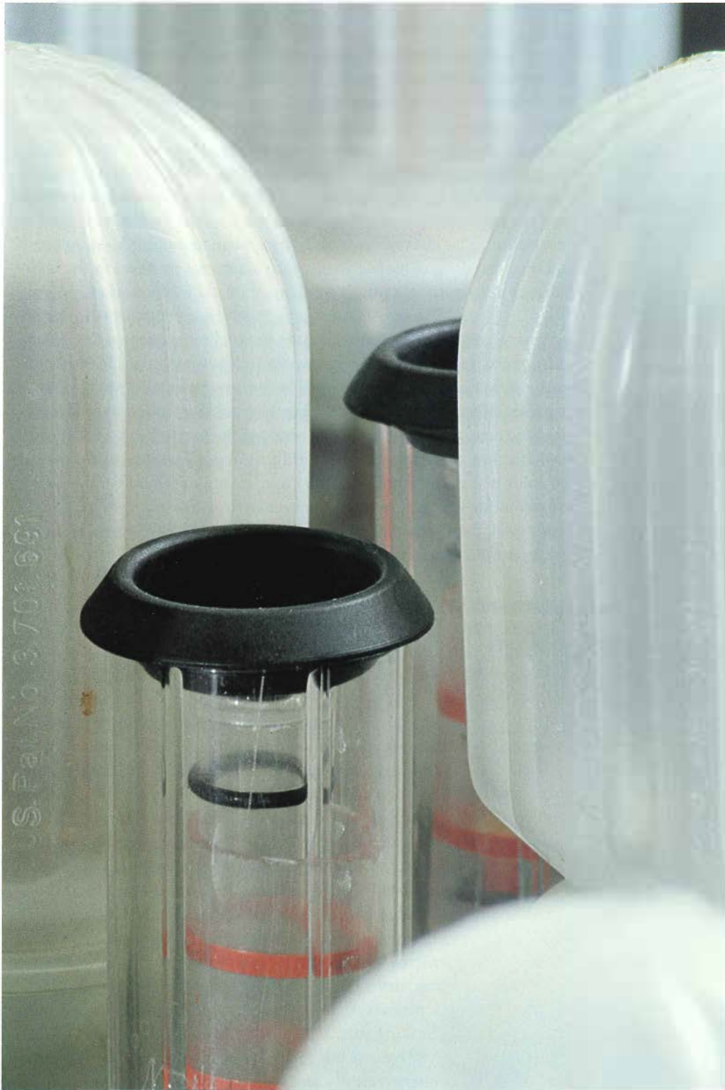
Hydrogen recombiners, part of a lead-acid battery used in testing advanced battery designs at EPRI's BEST Facility.
