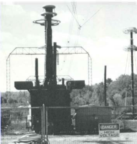
Methodical advance in electrical line design has been the role of the High-Voltage Transmission Research Facility since 1959. Texts and handbooks from the work are utility industry standards, and week-long seminars augment continuing research, which now covers the design of both ac and dc transmission facilities.
