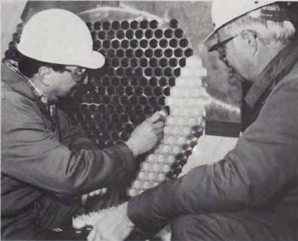
Figure 1 Foster Wheeler personnel installing explosive packages in a prototype tube bundle to demonstrate the simplicity of the procedure and its readiness for field applications.
