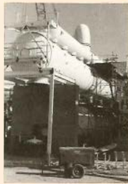
In the condensers, the hydrocarbon vapor is condensed to a liquid and cooled, then pressurized in the hydrocarbon circulation pumps and sent back to the heat exchangers for reheating.
