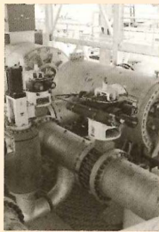
Inside Heber's special hydrocarbon turbine, the superheated hydrocarbon vapor spins the turbine that drives the 70-MW electric generator.
