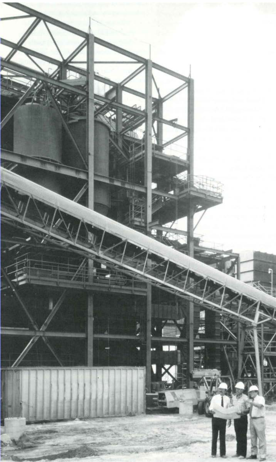
More than 40 small fluidized-bed boilers are being used for industrial applications in a number of industries. Shown is a Pyropower Corp. unit recently installed at California Portland Cement Co.'s Colton plant.
