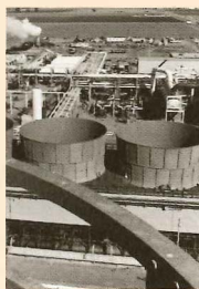
The nine-cell cooling tower reduces the temperature of the cooling water, which circulates in the two condensers at 140,000 gal/min (8830 kg/s), from 36 to 24°C (96 to 76°F).
