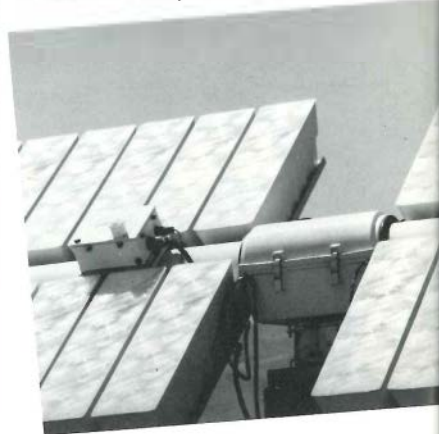
Concentrator array under test at PG&E
