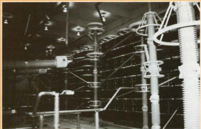
Thyristor valves at Comerford station, New England multiterminal project
