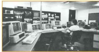
Network control center
