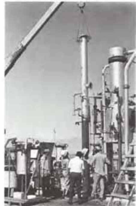
Figure 2 Installation of a steam-stripping column on the reboiler test unit at Cerro Prieto. The original 1000-lb/h upstream \text{H}_2\text{S} removal test unit is on the right. The stripping module increased removal efficiencies for \text{H}_2\text{S} and \text{CO}_2 to 98% (from 94%). It also prevented the decrease in gas removal efficiency that had previously occurred at low vent rates. The vessel mounted in the frame in the left foreground is a catalytic reactor that was tested earlier in the project. The reactor is a way to treat the vent gas stream, which contains the \text{H}_2\text{S} removed from the main steam flow. The reactor achieved conversion efficiencies up to 97%, converting \text{H}_2\text{S} to elemental sulfur and other oxidized species.
