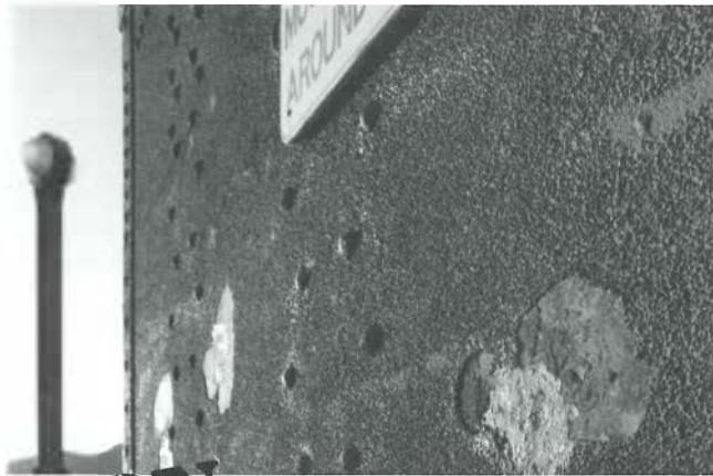
Common corrosion (Photo by Ron May)
