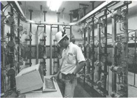
Monitoring systems relay room
