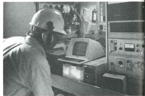
Flue-gas sampling and analysis system
