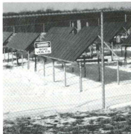
Detroit Edison's 4 kW of ECD Sovonics modules
