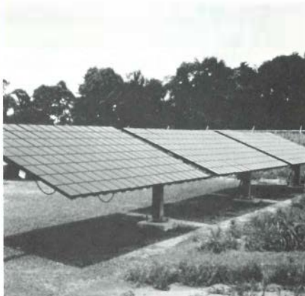
Philadelphia Electric's 8 kW of Solarex modules
