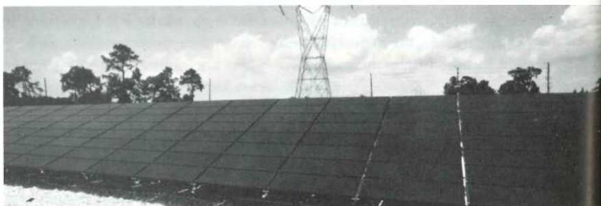
Florida Power Corp.'s 15 kW of ARCO Solar modules
