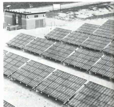
Alabama Power's 55-kW field of Chronar modules
