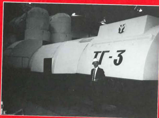
A supercritical district heating turbine at Moscow's station 26 reflects the Soviet commitment to the efficiencies of supercritical operation.
