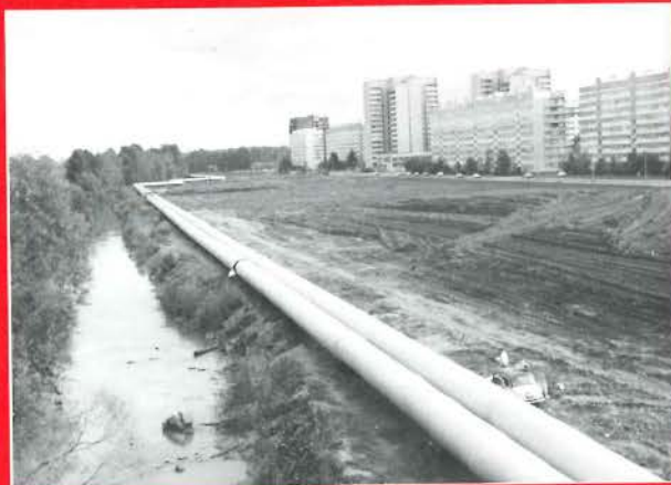
Five-foot-diameter pipes in Leningrad's district heating system deliver hot water directly to users in thousands of apartments; for scale, note the car parked next to the piping.
