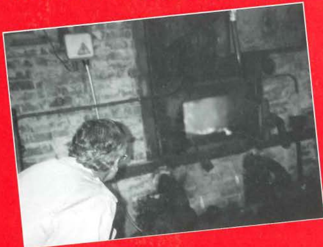
This 6-ton/hour bubbling-fluidized-bed test boiler at the Central Boiler and Turbine Institute's Barnaul facility is representative of new Soviet initiatives in emissions control.
