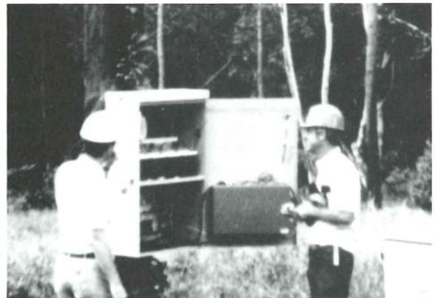
T&D sectionalizing switches
