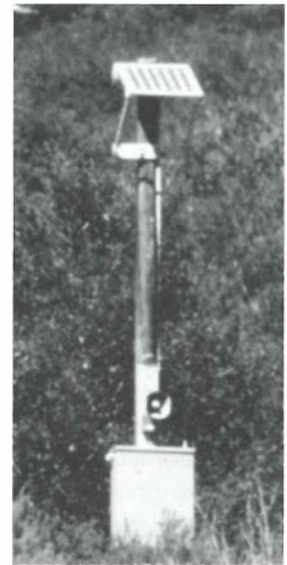
Power plant warning siren
