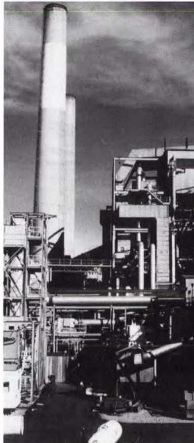
Arapahoe Emissions Control and Test Facility
