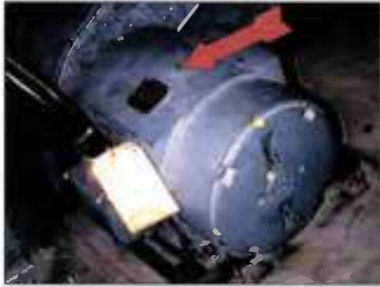
Typical hot spots on normally operating motor
