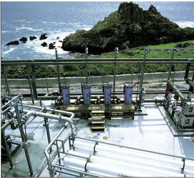
Reverse-osmosis units at Diablo Canyon nuclear plant
