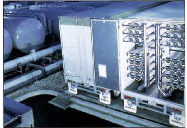
Santa Barbara, California, desalination facility
