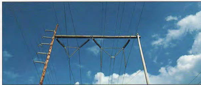
Low-field test lines at HVTRC (left to right: vertical split-phase, twisted-conductor, cruciform split-phase)
