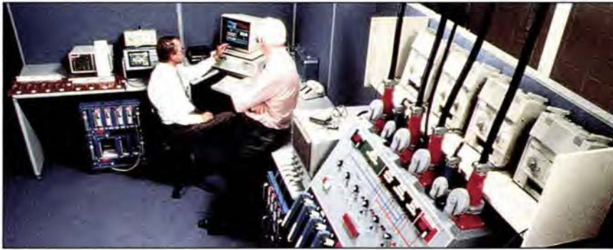
The Power Quality Test Facility features a wide variety of measurement and test equipment.
