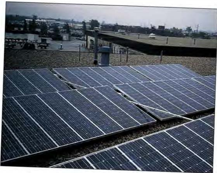
12-kW system at Wisconsin Public Service Corporation
