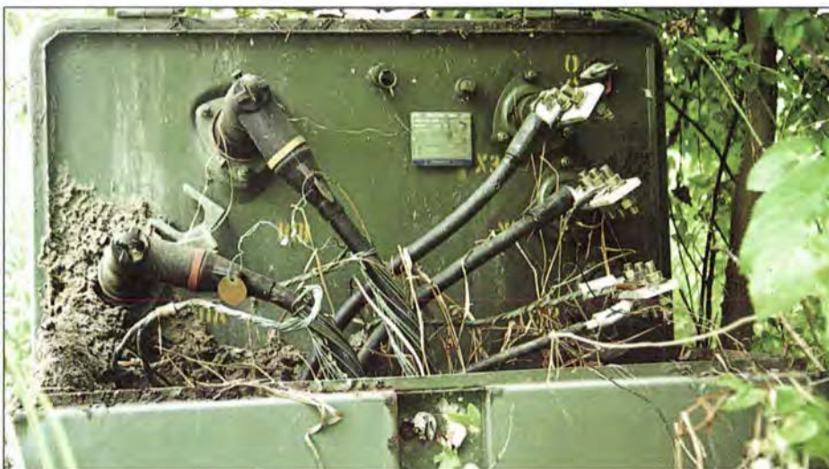
A fire ant mound clogs the interior of a residential transformer.
