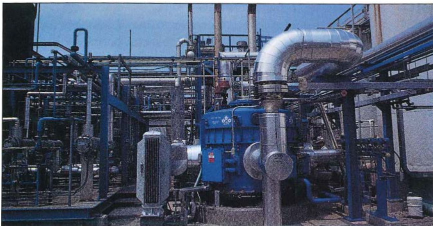
EPRI's modular fuel cell pilot plant at Destec's coal gasification test facility in Plaquemine, Louisiana
