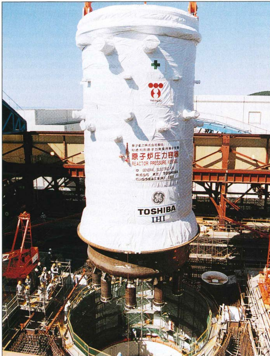
JAPAN GOES FIRST The world's first advanced light water reactors—based on General Electric's ABWR design—are now under construction at Tokyo Electric Power Company's Kashiwazaki-Kariwa site. The first of two 1356-MW units is expected to begin operation in 1996, less than five years after groundbreaking. Already licensed for use in Japan, the ABWR is being constructed under a joint venture agreement between GE, Hitachi, and Toshiba.
