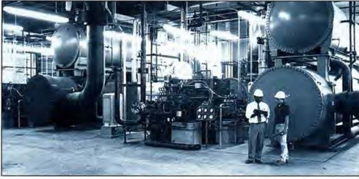
This chiller plant in downtown Indianapolis is part of a district cooling system run by Mid-America Energy Resources, a subsidiary of IPALCO Enterprises, the holding company of Indianapolis Power & Light.
