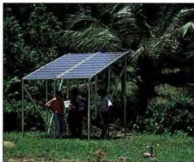
Photovoltaics powers a rural community water system in the Dominican Republic.
