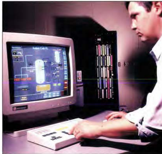
Digital control system display
