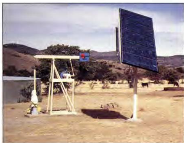
WEST TEXAS UTILITIES This PV panel powers a water-pumping system at a cattle ranch in west Texas. Under a joint venture agreement with Solamotor of Texas, WTU will install 20 such units over the next year.
