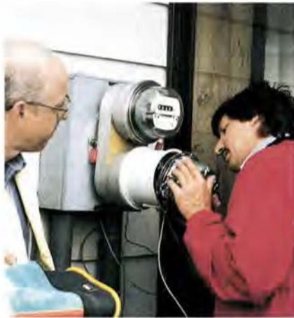
Installing a NIALMS recorder in Buckeye Power's service area
