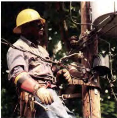
An RG&E line worker installs the net current control device beneath a distribution transformer.
