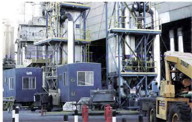
Two transportable pilot-scale pulse-jet fabric filters were installed at the Mohave station.
