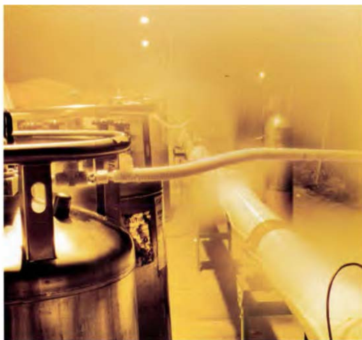
HTS cable testing in liquid nitrogen
