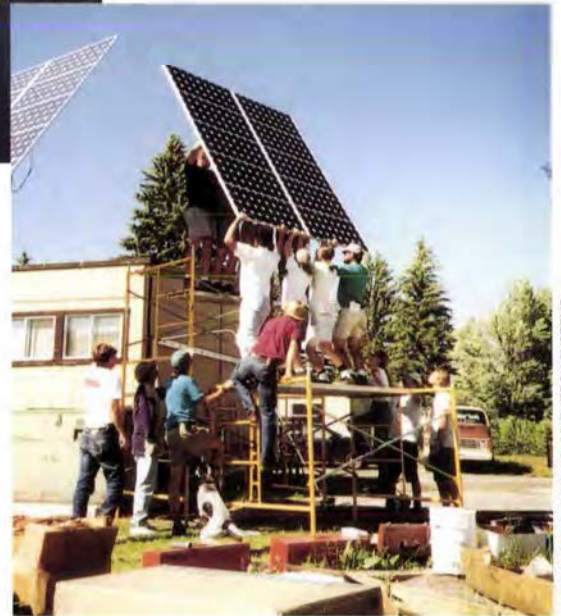
Volunteers install a 1.5-kW PV system at the Carbondale, Colorado, middle school. The project was funded by customer payments to Public Service of Colorado's Renewable Energy Trust.
