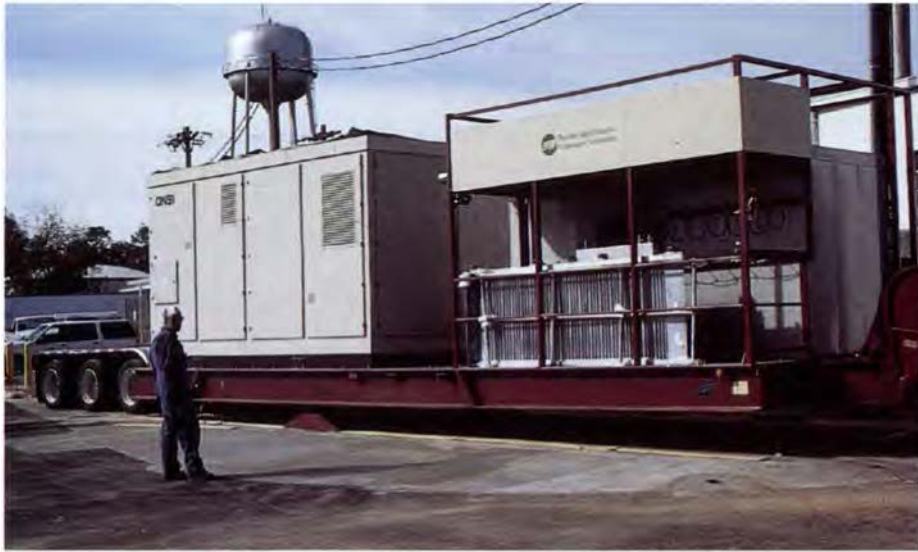
The traveling fuel cell being installed at a baby-clothing manufacturing plant in Jackson, Georgia.
