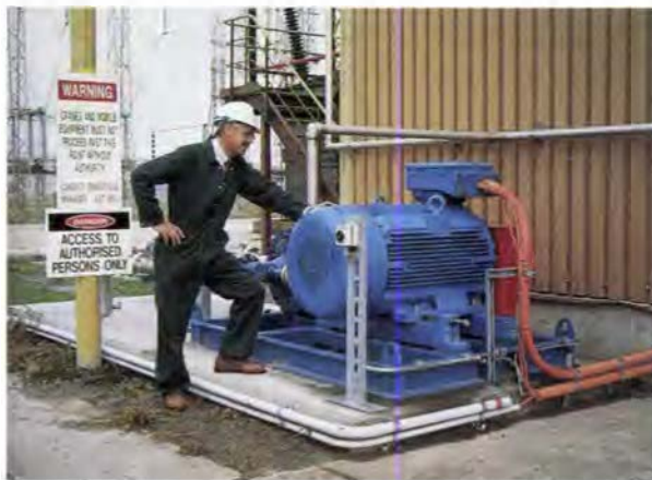
Spray cooler water pump at the Jeeralang station
