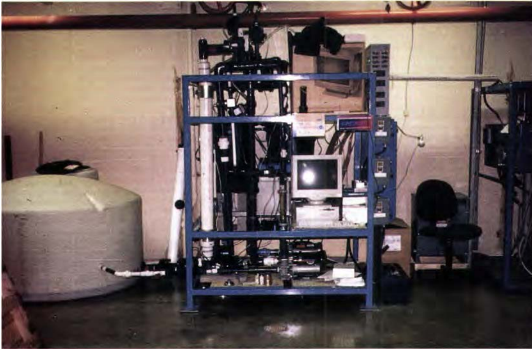
Pilot-scale membrane filtration system in Decatur, Illinois
