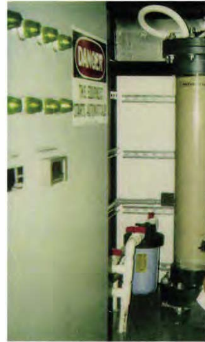
Inside EPRI's ion exchange trailer
