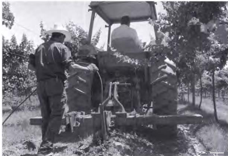
Water lines are buried at root level in research on subsurface drip irrigation (SDI) at California State University at Fresno. Computer-controlled SDI systems with electric pumps are expected to use 25–50% less water than conventional irrigation approaches.
