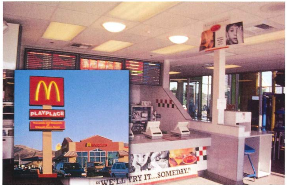
Daylighting controls were installed in this McDonald's restaurant near Pittsburg, California. The fast-food chain is considering offering such controls as an option for new franchisees.
