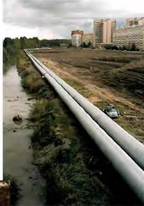
Large-diameter hot water pipes in St. Petersburg, Russia
