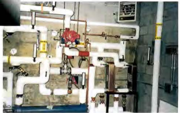
Hot water customer service connection in Jamestown, New York
