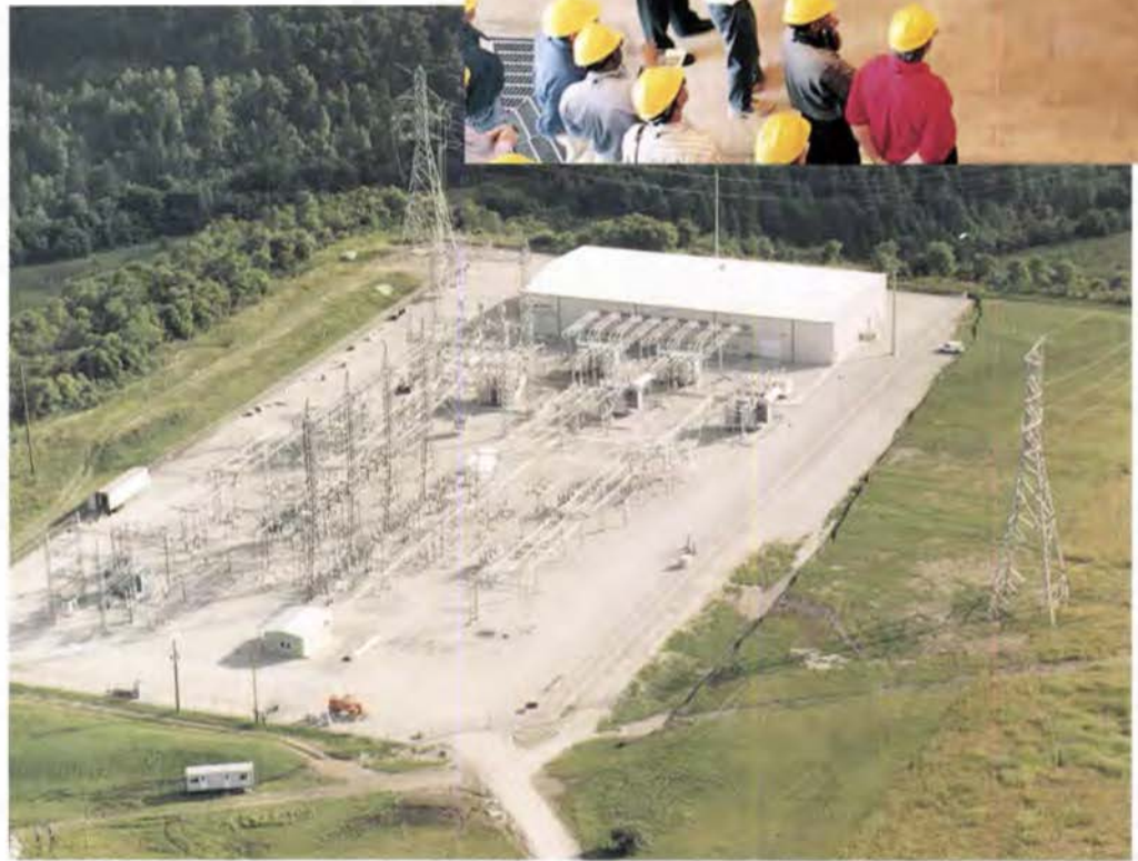
AEP's Inez substation
