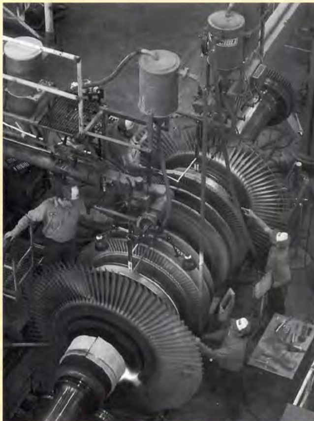
Rotating parts—turbine rotors, disks, and blades—are among the most critical and highly stressed components in nuclear and fossil power plants. EPRI provides technical assistance and on-site troubleshooting for these and other components through its Repair and Replacement Applications Center.
