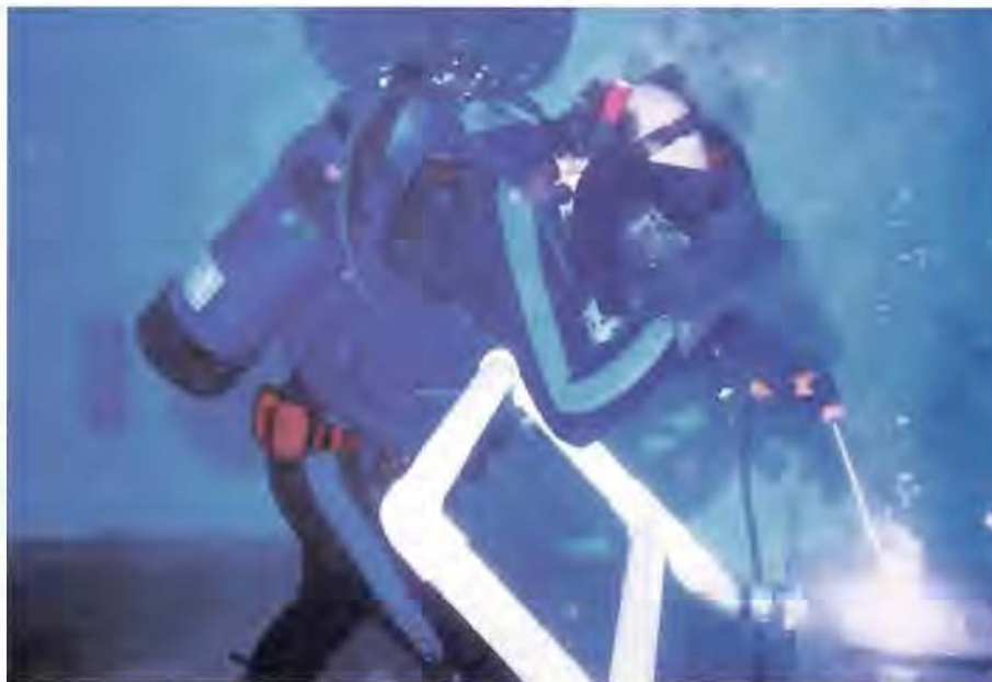
EPRI innovations in underwater welding have resulted in better arc stability, splatter-free welds, and improved worker safety. Used for repairs at nuclear plants, underwater techniques are safer for welders, since the water provides a degree of radiation protection. And for repairs without divers, an automated underwater method based on flux-cored arc welding has been developed.
