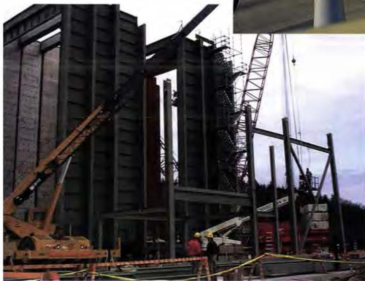
COURTESY PG&E GENERATING
