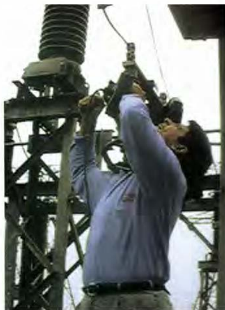
The South African utility ESKOM successfully used the GasVue leak detection system on energized equipment at two gas-insulated substations and two outdoor substations.
