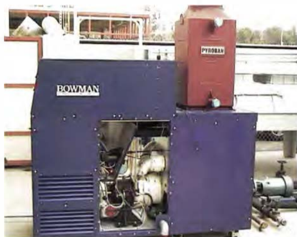
This 45-kW Bowman microturbine was installed for cogeneration at a University of California, Irvine, laboratory. Cosponsoring the project with EPRI are Edison Technology Solutions, DOE, and the California Energy Commission.
