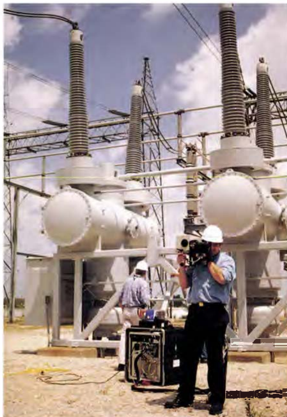
Illinois Power, one of two dozen utilities that have hosted GasVue demonstrations, used the system to test for SF 6 leaks from circuit breakers and other energized equipment at its Clinton substation. In an economic comparison with conventional bubble testing, the utility documented savings of $12,000 in avoided costs in just this single GasVue application.
