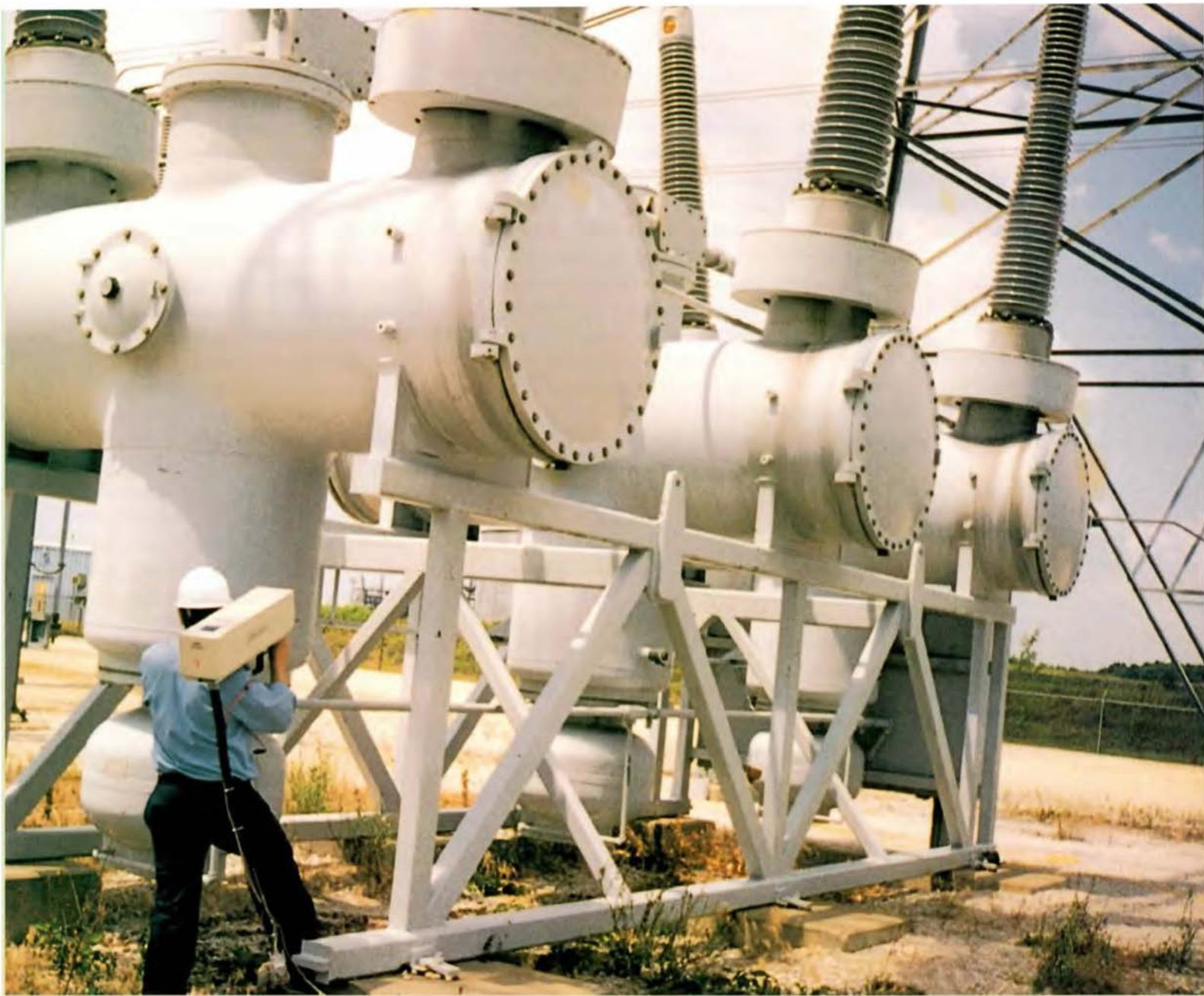
The GasVue camera can be used to inspect substation equipment, like this 500-kV SF 6 -insulated circuit breaker, while the equipment is energized.
