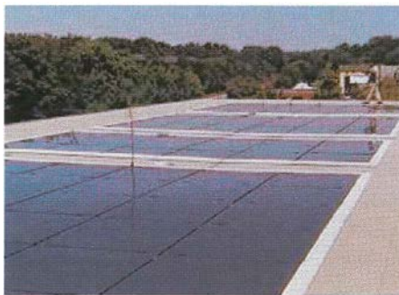
13.2-kW (ac) system using Atlantis PV modules, installed by New York Power Authority on a community center in Tuckahoe, New York.
