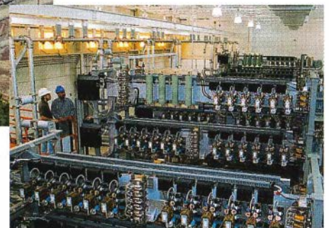
Banks of gate-turnoff thyristor control valves are the electronic heart of the CSC.
