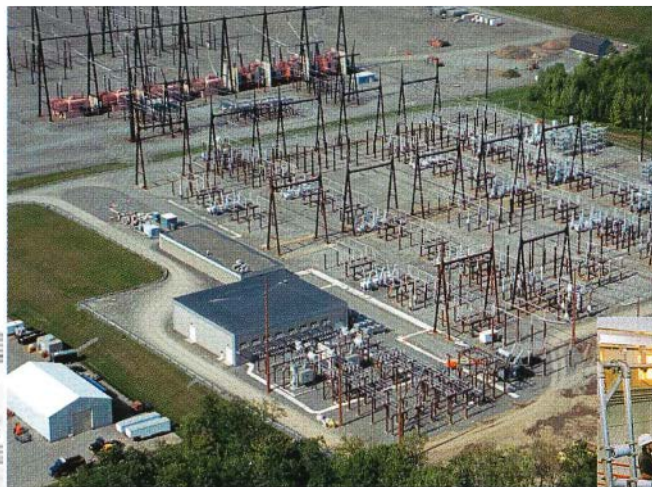
Aerial view of NYPA's Marcy substation; CSC is housed in larger building, left foreground.
