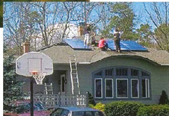
This is a 1.6-kW (ac) system using AstroPower PV modules, installed by GPU Solar in Lakewood, New Jersey.
