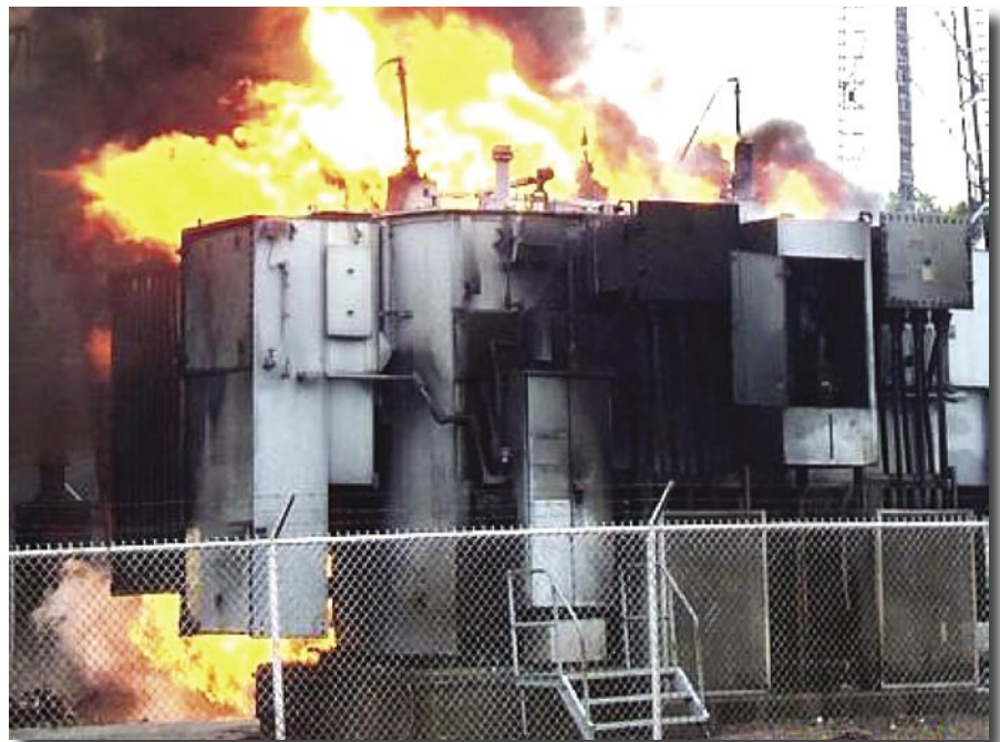
Modern-day security threats can be both physical and cyber-based. An intruder could destroy a substation transformer with a bomb or by setting a fire, but a computer hacker could accomplish the same end by sending the transformer overload signals, causing it to rapidly overheat and explode.
