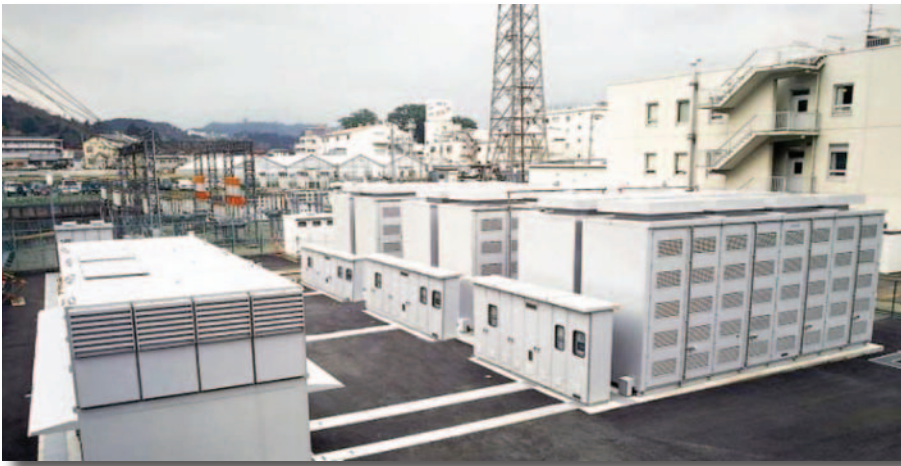
Sodium-sulfur batteries, offered commercially under the trade name NAS, have shown great promise for utility applications in the 1–6-MW range. Based on a high-temperature reaction between sodium and sulfur, the NAS battery features excellent stability, robust cycling, and minimal on-site maintenance. Shown is a 6-MW unit installed at a substation in Ohito, Japan.
