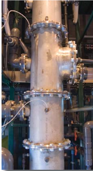
Lab-test absorber tower
