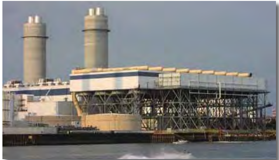
Dry cooling has obvious advantages in water-constrained regions but may be a good choice elsewhere as well. For example, the Mystic generating station on Boston Harbor chose a dry system over once-through cooling to avoid concerns over possible impacts on aquatic life.
