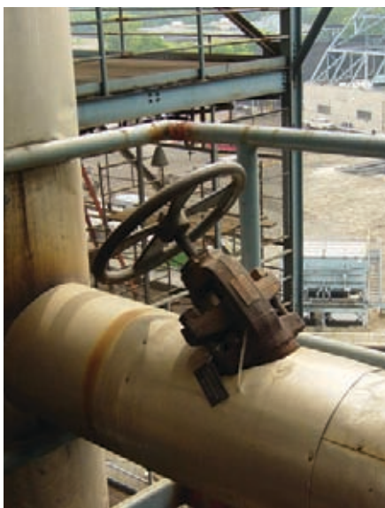
Designs for new facilities often fail to adequately consider ergonomics and maintenance access. This valve could easily have been re-oriented in the design stage to face the worker.
