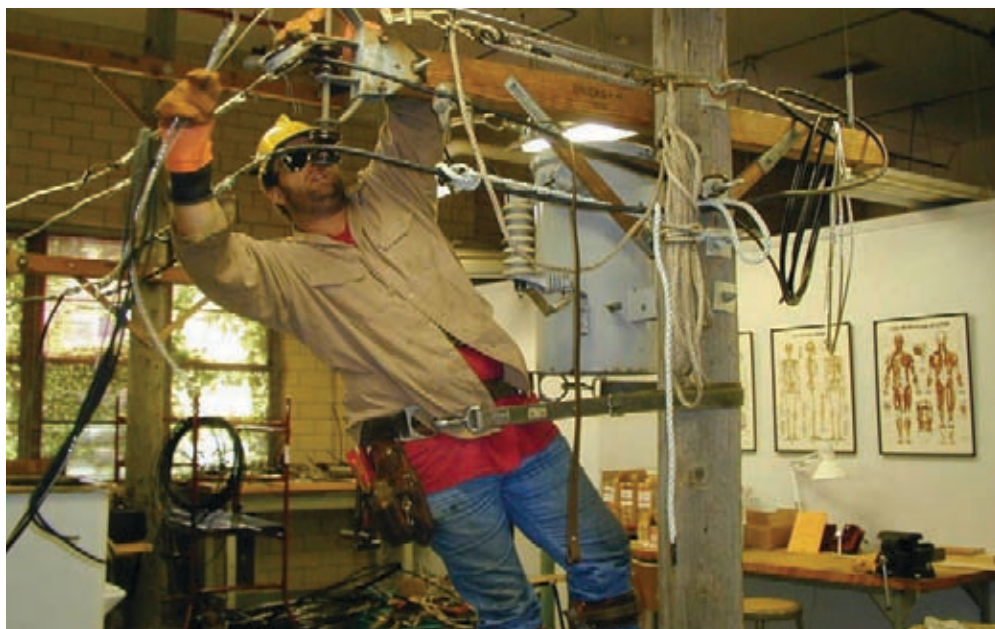
Musculoskeletal injuries—typically sprains and strains resulting from awkward body positions or movements—account for the largest class of utility injuries. Ergonomic studies in the field and on full-scale mockups in the laboratory have identified specific causes and solutions, which are outlined in EPRI's series of ergonomics handbooks.
