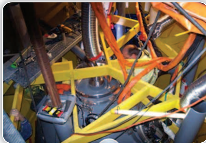
Workers can practice their techniques in full-scale mockups of high-radiation areas, reducing their time in the reactor environment.
