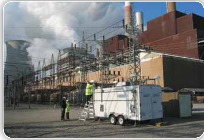
Disk-cone antennas on the corners of a trailer detect radio-frequency emissions that indicate the location of deteriorating substation equipment.
