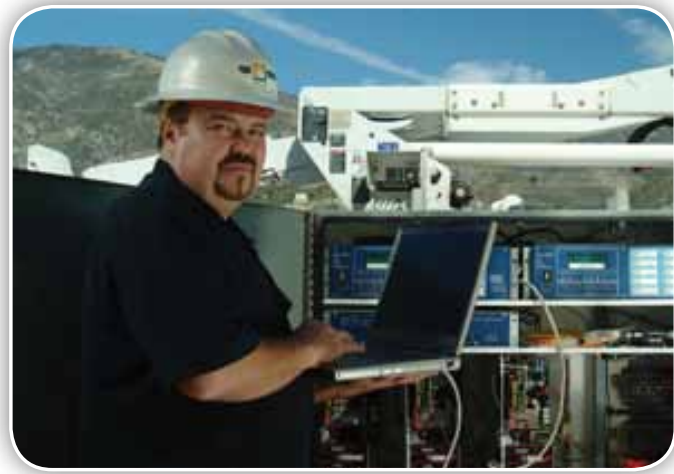
A technician tests the remote control interrupters on SCE's Avanti advanced distribution circuit.
